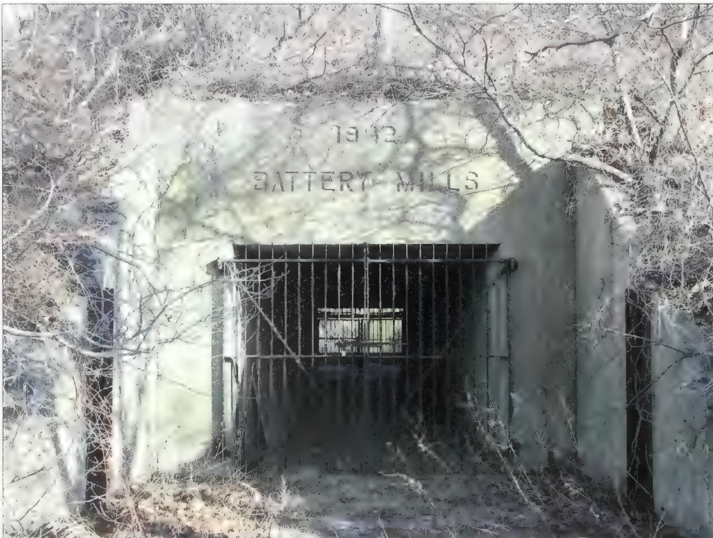
Figure 5.90. View looking east at a bulkhead entry, Battery Mills. All woody vegetation growing on or within four-feet of concrete features like the bulkhead entries should be removed (Olmsted Center, January 2009).
